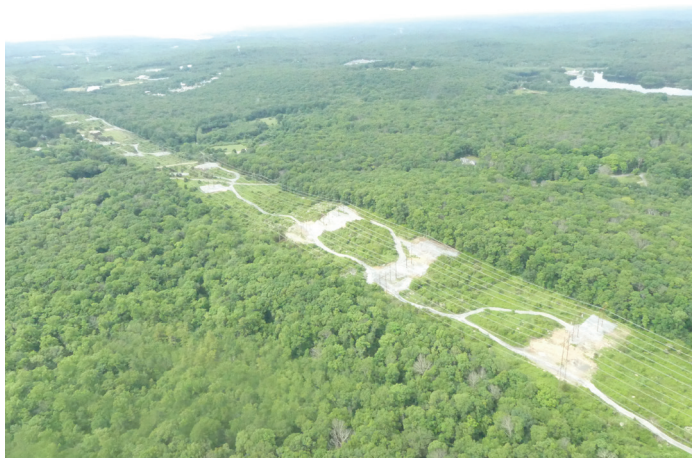
The new packed gravel access roads and pads on a right-of-way. Photo: CBS.
